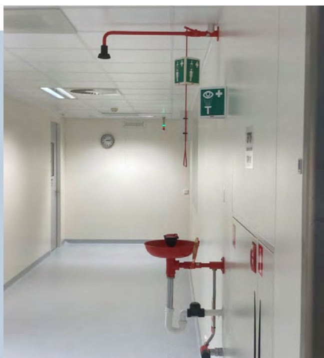
Figure 13-4: A shower and an eye shower in a pharmacy of a hospital (for emergency purposes in case of an incident) at the Meander Medical Centre, The Netherlands
